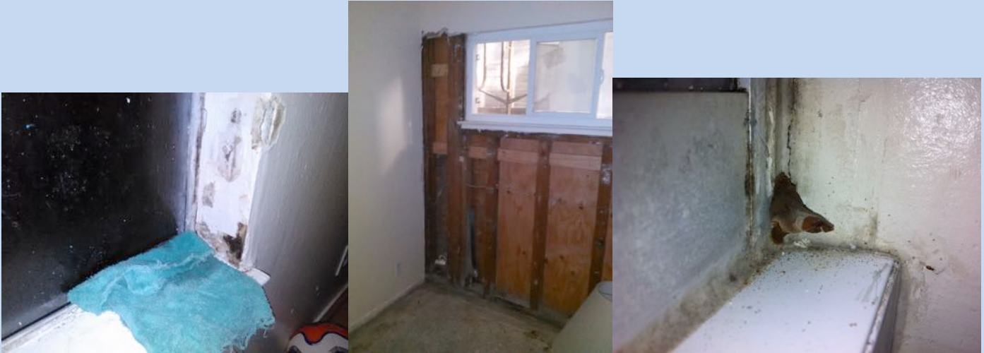
475 ALCATRAZ: WATER DAMAGE, EXPOSED WALL STUDS, AND MUSHROOMS! ↑
